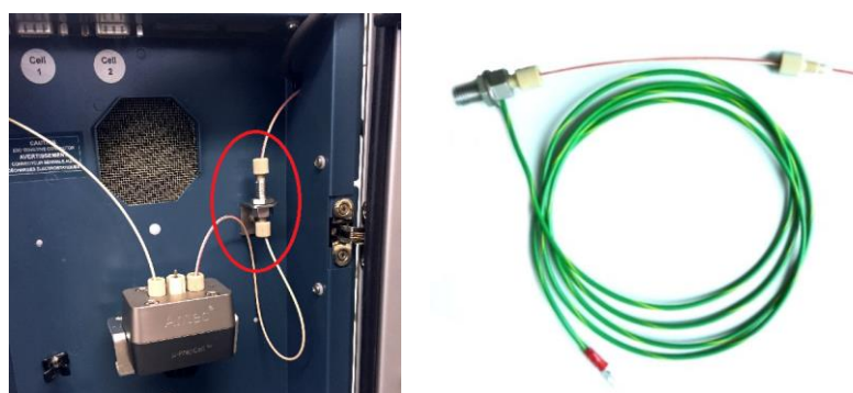
Fig. 5. The grounding kit inside the ROXY (left) or for external use (right).
